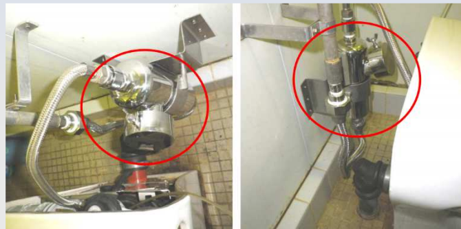
Unit fitted in toilet onboard
